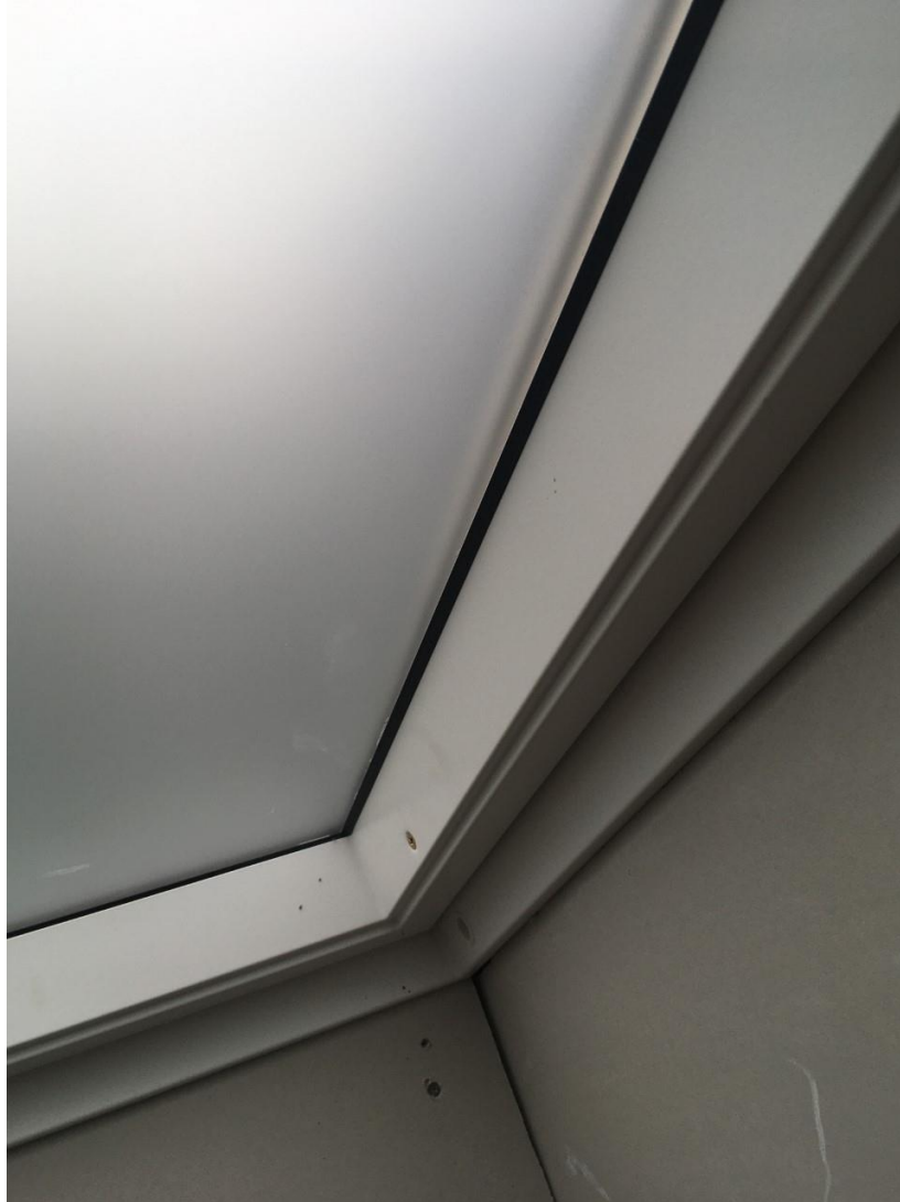
Figure 2: Roof lights currently screwed shut and obscure glazed
