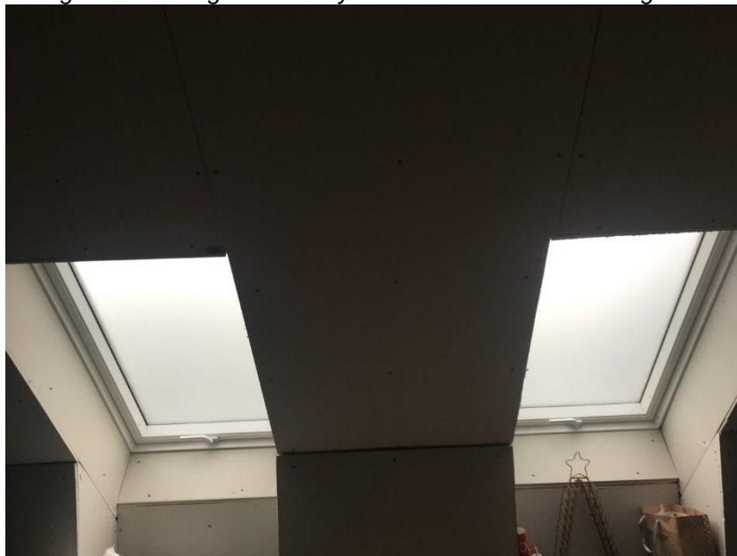
Figure 3: Both roof lights serving the loft area obscure glazed
